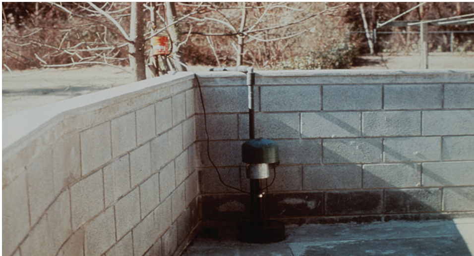
Figure 8-6. Small patio floodwall with sump pump.
