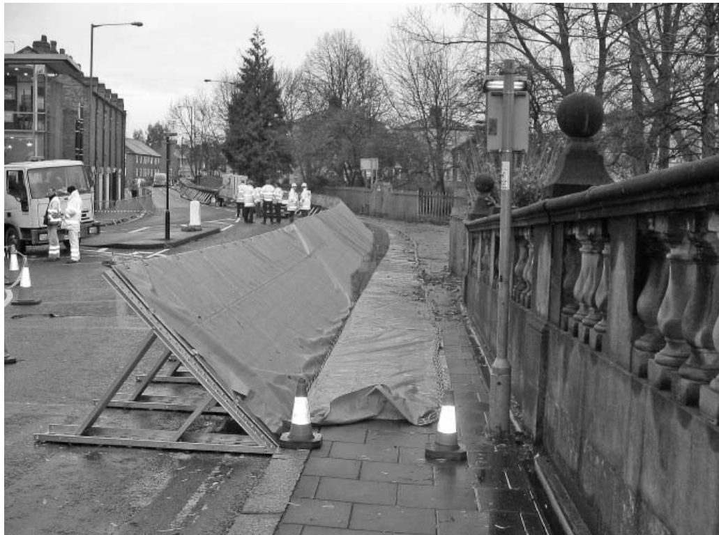
Photo 3.15: temporary flood barrier deployed. Source: J Lamond
