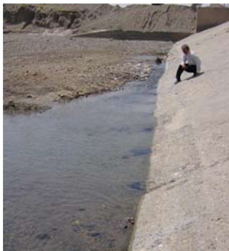
Figure 3: Water emerging from weepholes
