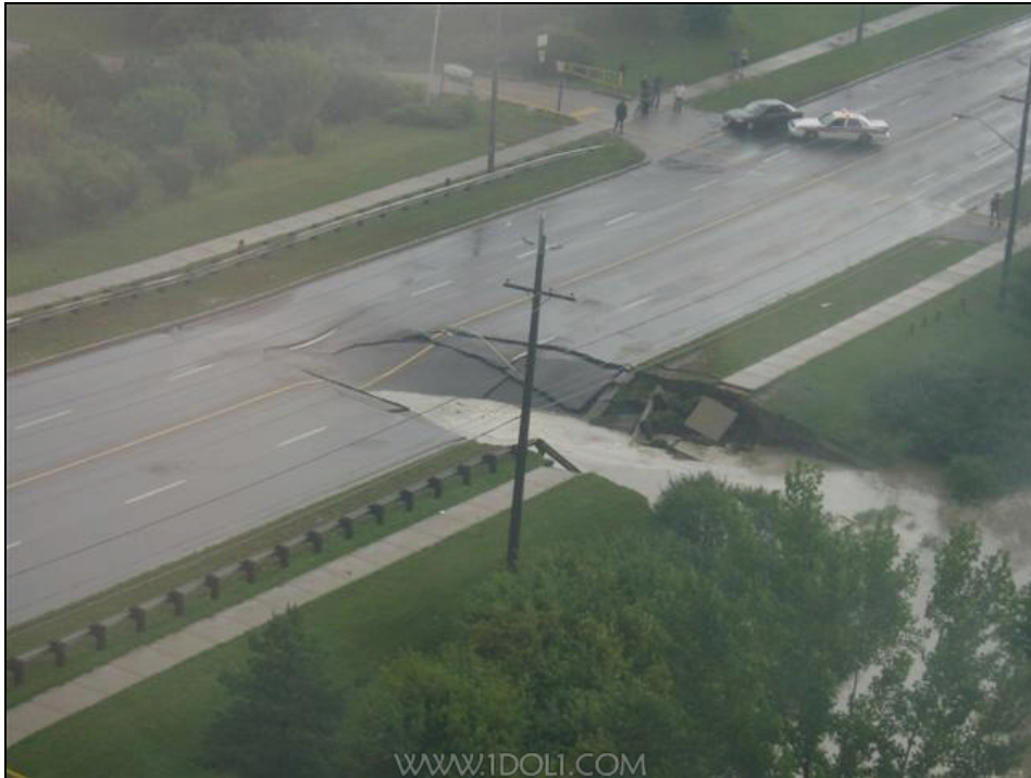
Photograph 9.3: Failure of a road surface due to “piping”, occurring around the culvert
