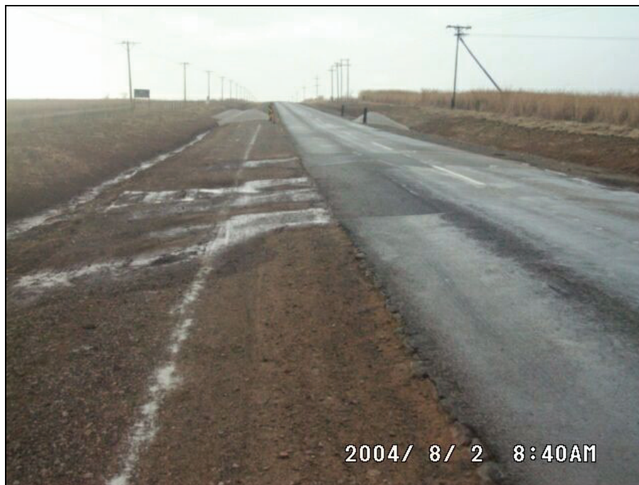
Photograph 9.1: Typical conditions associated with poor sub-surface drainage design
