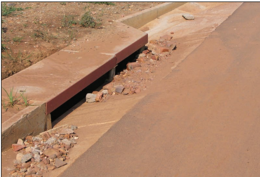
Photograph 5.2: Kerb inlet with deposited debris (side outlet)
