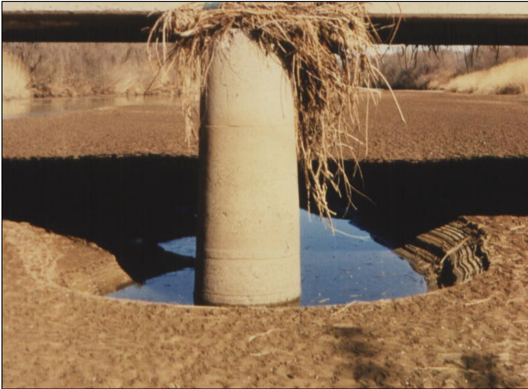
Photograph 8.3: Local scour at pier
