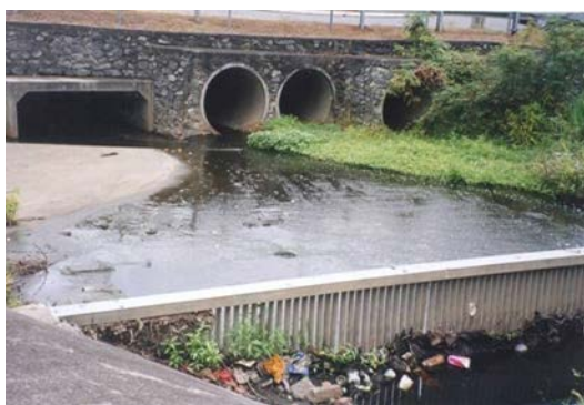
Figure 7.5.3.1(a) – Trash rack
