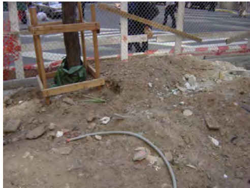
Example of inadequate tree protection
