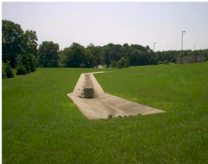
Figure 9-25. Existing sinkhole-plagued detention basin.
