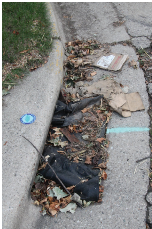
Figure 9-7 Example of a Neglected Catch Basin.
