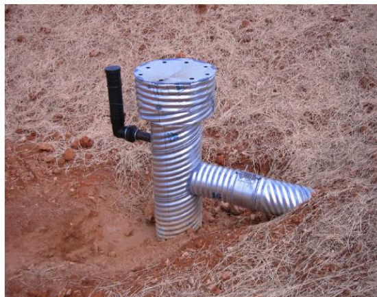
Figure 7.31-6 Dewatering device on Riser with Trash Rack
