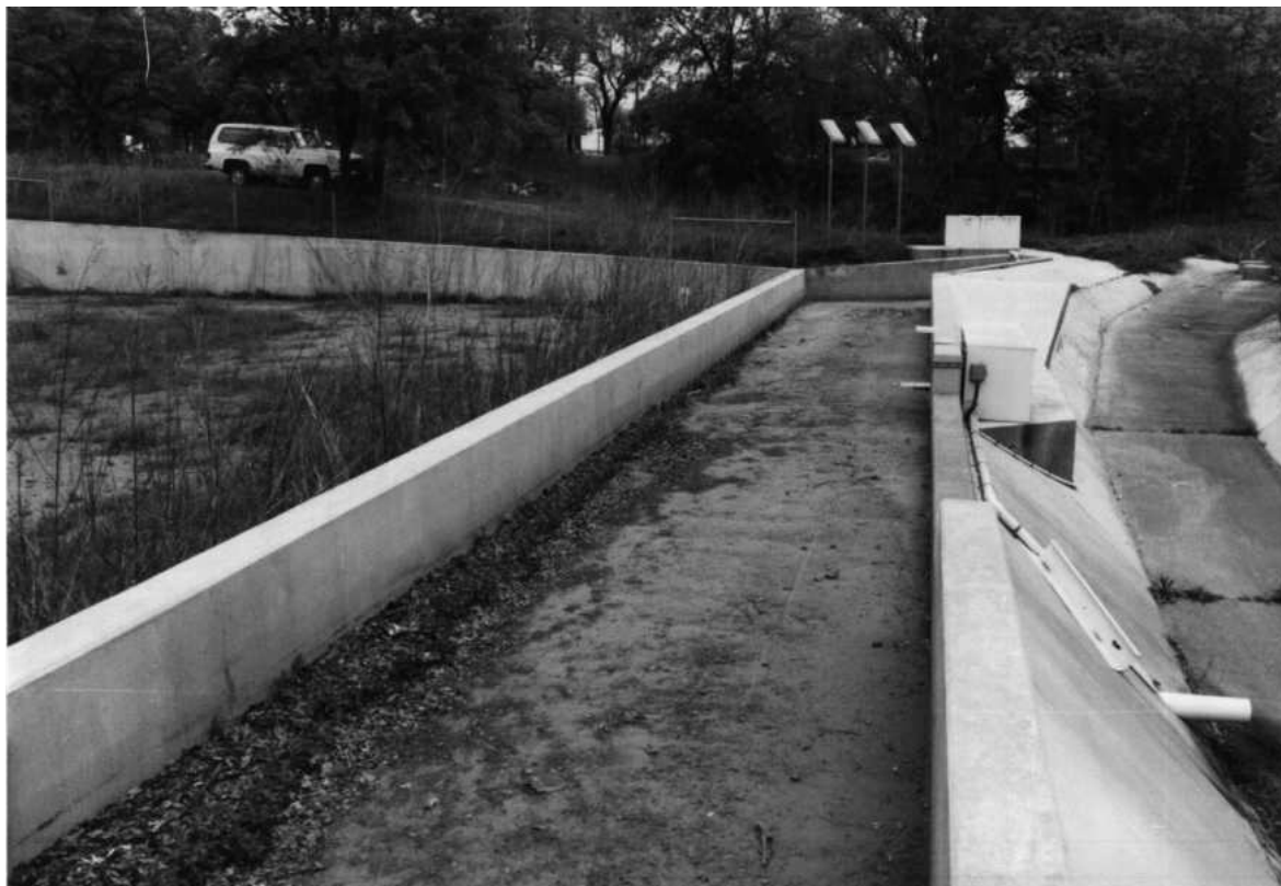
FIGURE 3.12C - 2 Sedimentation Basin of Jolleyville Partial Sedimentation System
