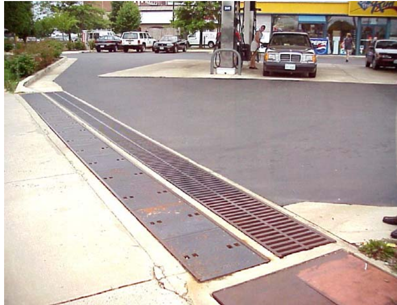
Sand Filter at entrance to service station.
